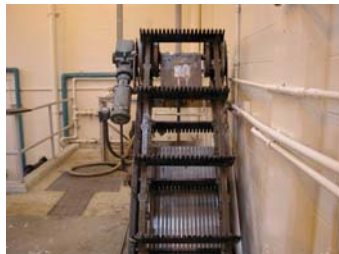
The Main Plant Location Duperon FlexRake
