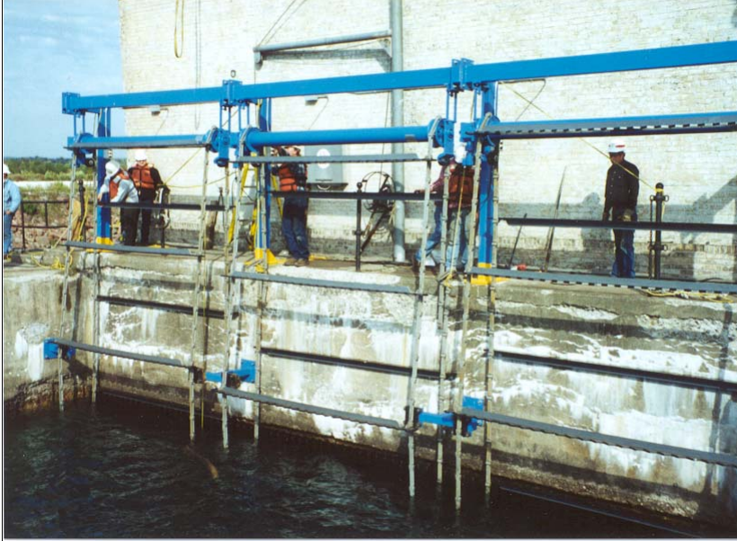
St. Mary's Falls—USACE Hydroelectric Plant
