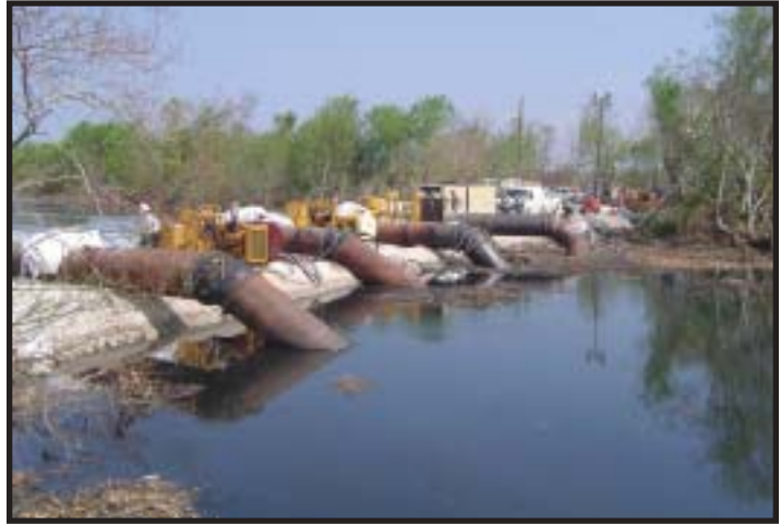
Four 42" Hydraflors, each capable of 70,000 gpm, at the Pump Station 15 Canal pump out Hurricane Katrina floodwaters.
