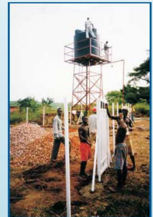
Community members setting up a fence and overhead tank for the SolarPedalflo.
